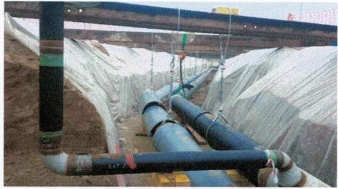
Tipping of pipes to replace
