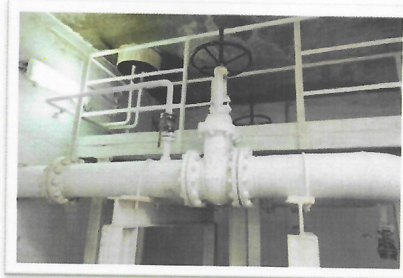
View of high point valves room
