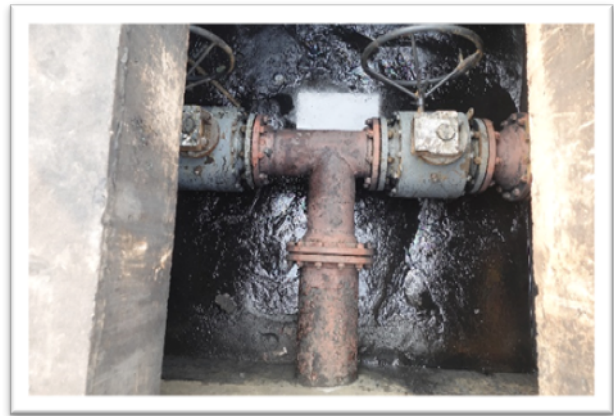
View of hydrant chamber
